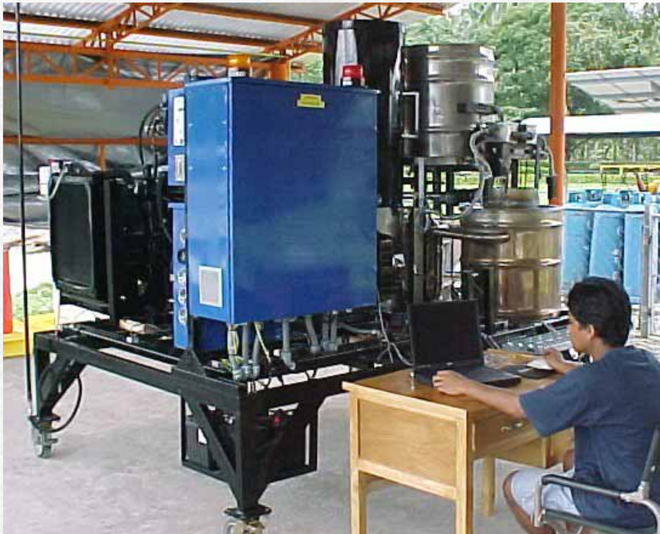
Community Power Gasifier: 12.5 KW
